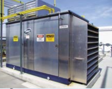
◀ Pictured is a 200 hp non-lubricated CNG compressor package with acoustical enclosure.
