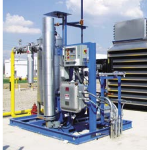
Pictured is a single tower dryer with on-skid regeneration. Dryers reduce the moisture content of the gas.
